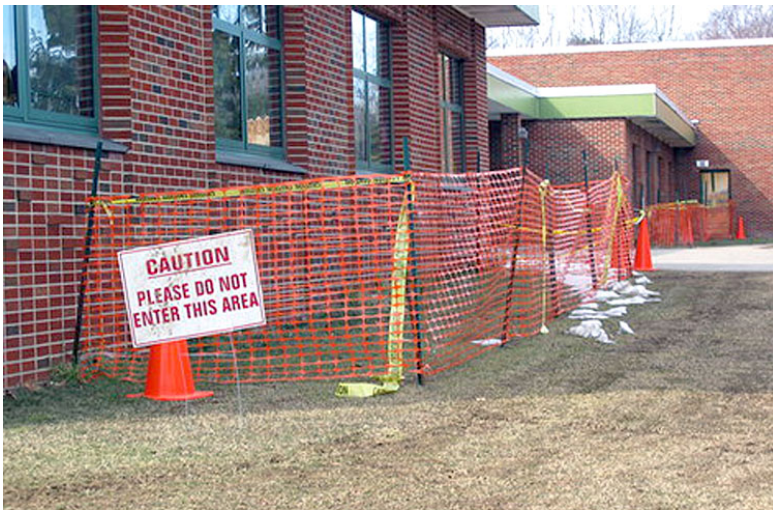
Monsanto marketed PCB-based caulking to schools and other municipal buildings throughout the U.S beginning in 1950, touting the chemical's ability to contract and expand with changing temperatures. Studies suggest that any school built or renovated between 1950 and 1977 may contain PCBs. Photo credit: pcbinschools.org
