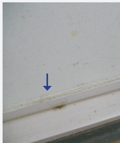
FIGURE 1 PCB-containing caulk along the building envelope of a school.
